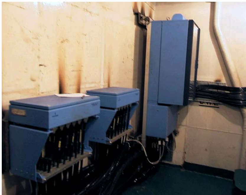
Figure 2 - The Transceiver Unit and TX Junction boxes on "Bligh".
