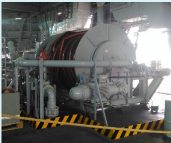
Astern Reel Main Drive Motor
