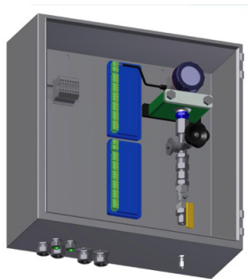
Figure 7: Temperature- and pressure transmitter cabinet installation
